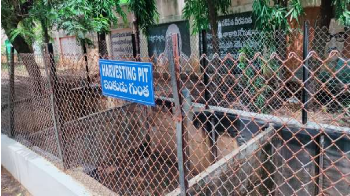
Rain water harvesting pit opposite to sports complex
