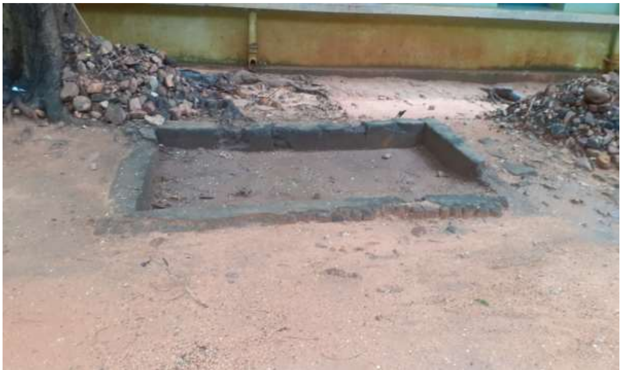
Rain water harvesting pit at western side of Electronics Dept
