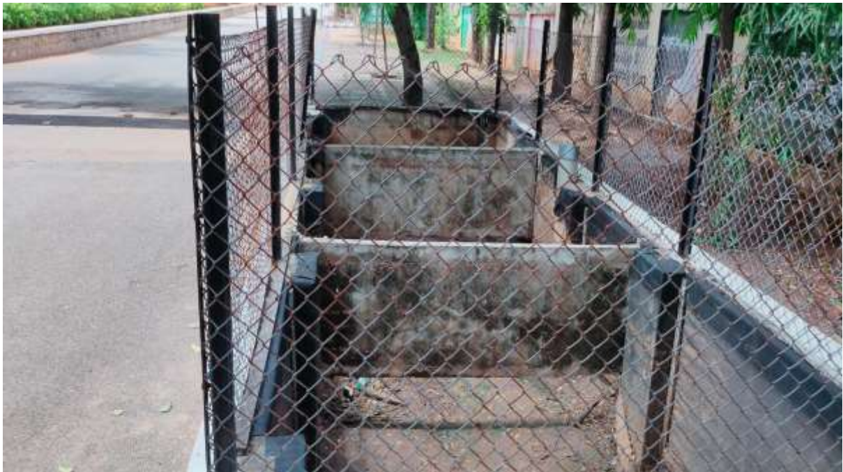
Rain water harvesting pit in front of the sports complex
